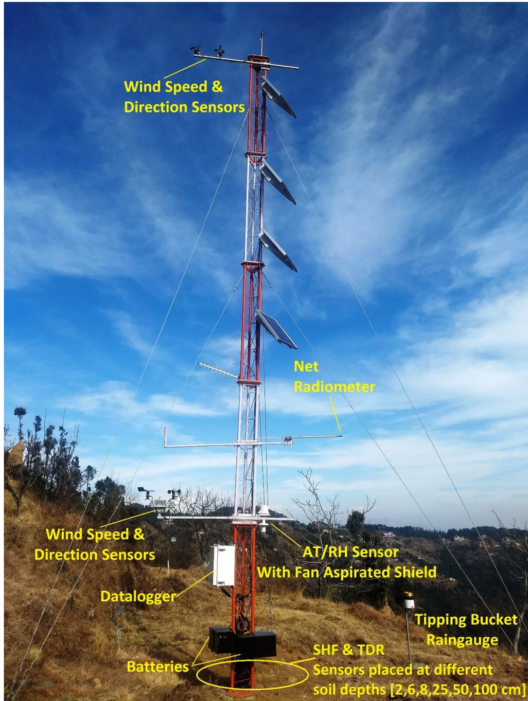
Fig. 3. 4 The automatic weather station (AWS) installed at Kanataal
